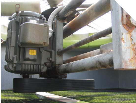
Before: Cooling tower fan with 5 strand V-belt drive.
