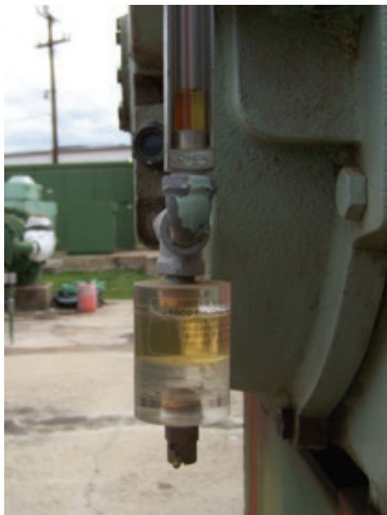
Figure 14: An oil sight glass (bottom sediment and water bowl) installed on a drain is a great indicator of problems such as water ingress or degraded oil.
