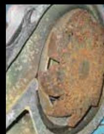
Suspended Debris in Coolant
