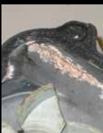
Deposits /Calcium Buildup
