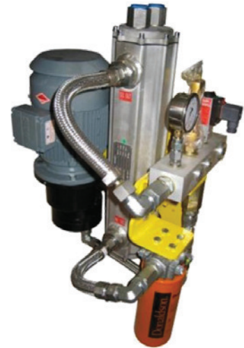
Gearbox lubrication system.
