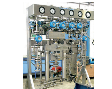
Filter station for the filtration of gases with STAUFF 3-way-selector ball valves for 250 bar / 3600 PSI and +200°C / +392 °F.
